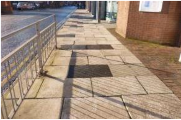
Photograph 24: Poor Quality Surface of Paving Slabs with Areas of Tarmac
