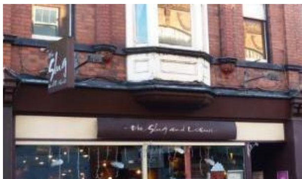
Photograph 30: Intrusive wiring to 31-33 Stamford New Road
