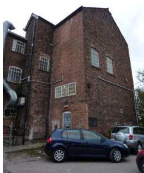
Photograph 28: Rear elevation of C.W. Bonson's Store Rooms in poor condition
