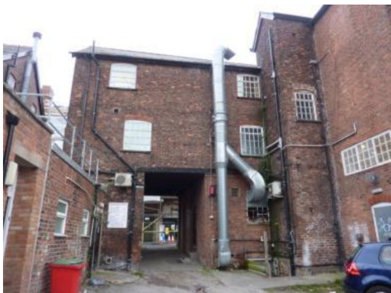
Photograph 27: Inappropriate ventilation system
