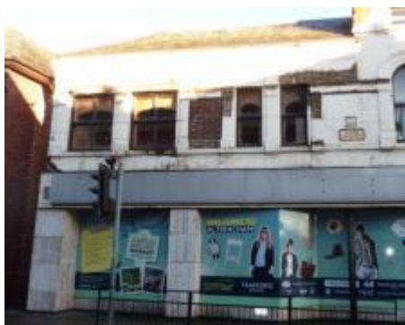
Photograph 29: Vacancy and decay to the upper floors on Cross Street
